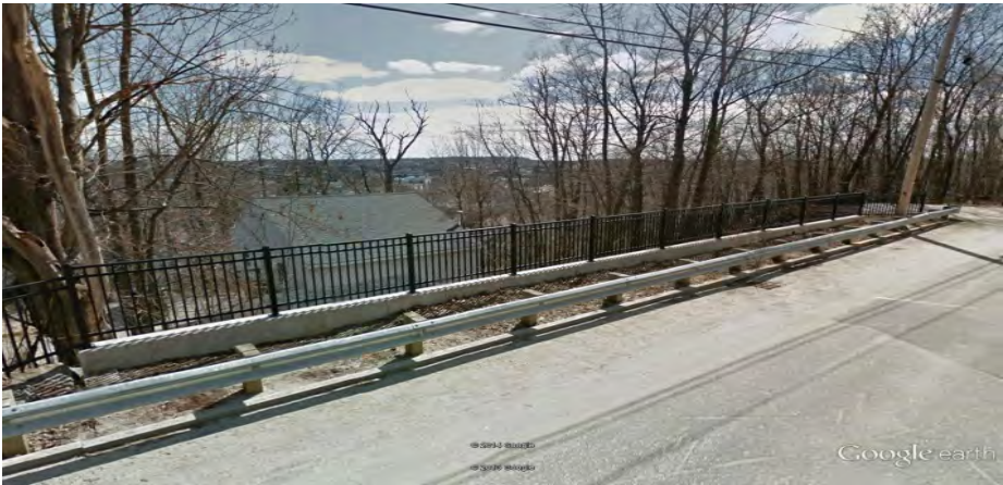
77 Highland Avenue – Reinforced concrete wall was constructed to replace a stone retaining wall in 2006.
