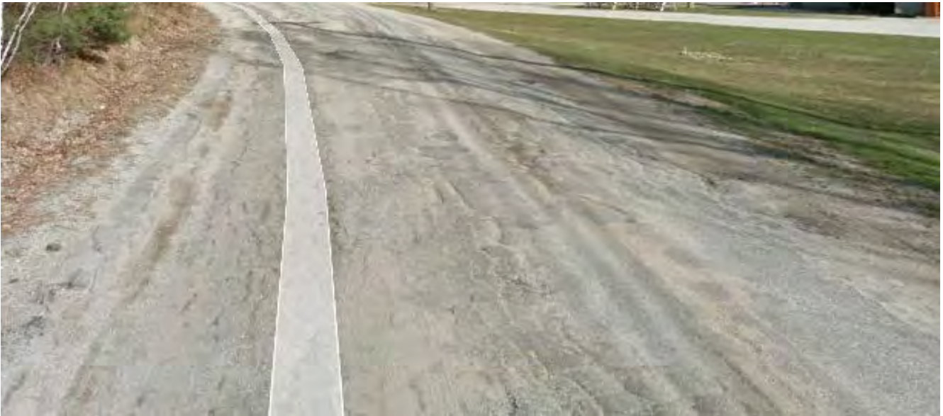
Summer Street (3000 lf) from Park to Mount Auburn – The roadway has a PCI rating of 37.58. The roadway will be converted to a one way in-bound with a turn-around outbound after the last driveway. The estimate for the reconstruction is $400,000.
