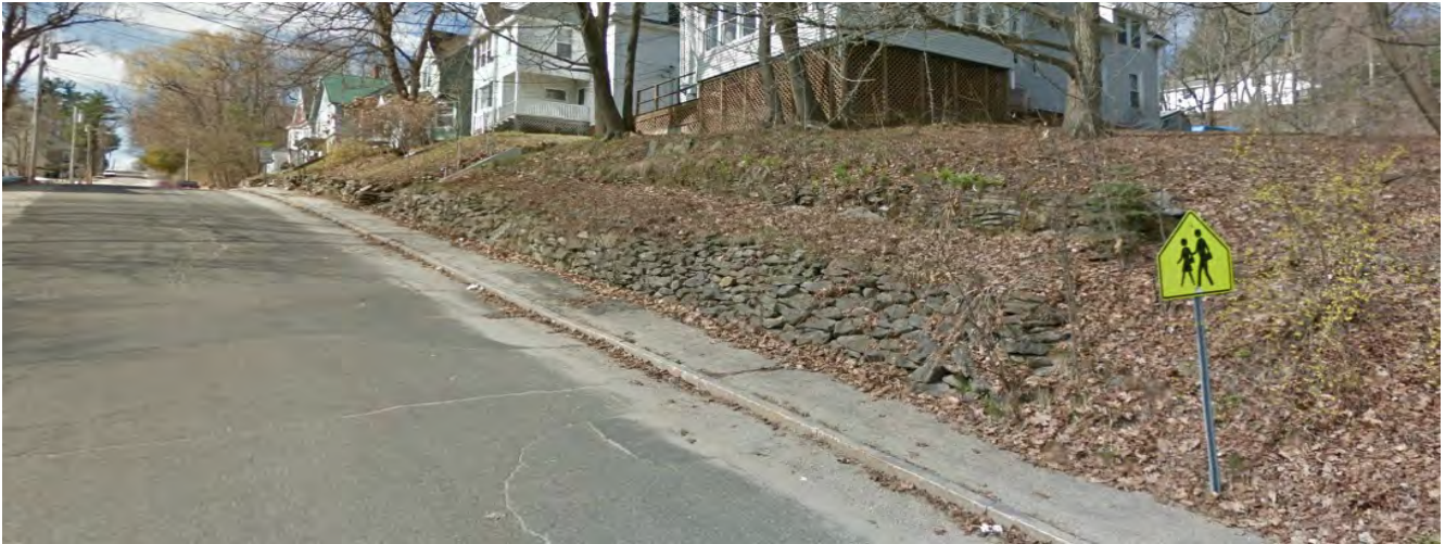
21 to 25 Western Prom – The original construction is uncertain. In 1969-70, the City reconstructed the wall as part of installing underdrain under the sidewalk on the northwesterly side of the street.
