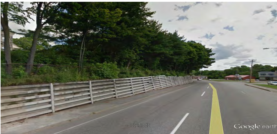
Minot Avenue Rotary – Metal bin wall constructed in 1957. A Maine DOT and City project will be replacing the bin wall in 2014.
