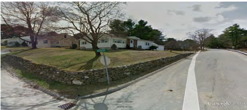
Vickery Road, starting at Riverside Drive – Dry stack stone wall repaired in 2004.
