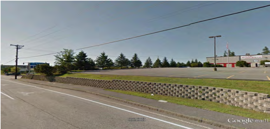
Mount Auburn Avenue along BJ's parking lot – Keystone Block wall constructed in 2001.
