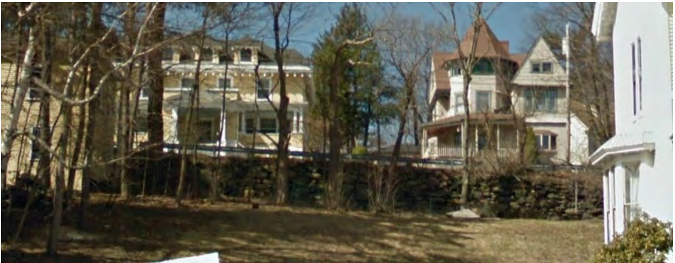
*Opposite 32 Beacon Ave – This wall was constructed by the City sometime after May 6, 1912 after approval of a petition to the City for a bank wall on the east side of Beacon St from Western Av to the angle in the street. *In FY15 CIP
