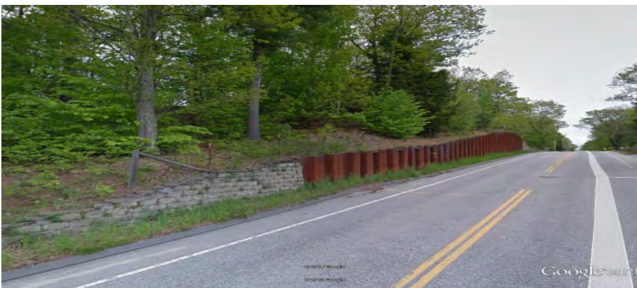
East Hardscrabble Road, across from David Drive – Sheet pile and block wall constructed in 1999.
