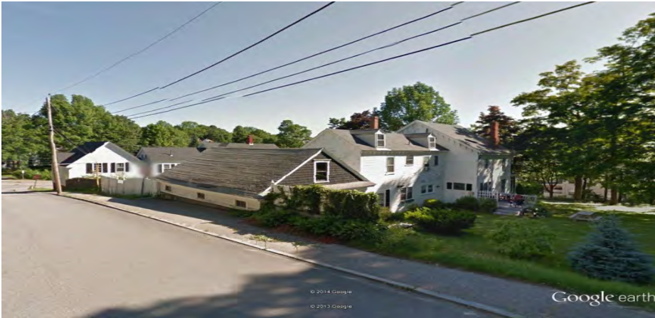
Forest Avenue at 7 Prospect St – Reinforced concrete wall was constructed to replace a stone retaining wall in 1995. The wall partially supports a garage.
