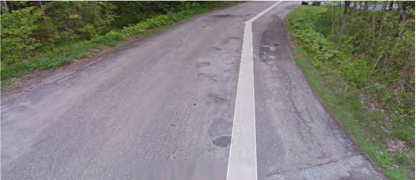
Valview Drive (7500 lf) from Garfield to dead end – The roadway has a PCI rating of 41.08. The estimate for the reconstruction is $1.25 million.
