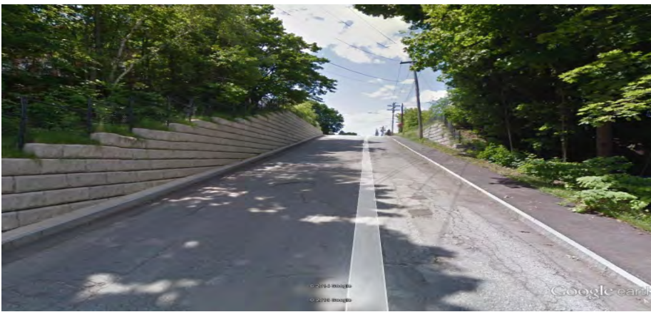
Dunn Street, both sides between Riverside and Second – Block wall constructed in front of pre-existing concrete wall in 2010.
